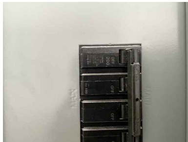
Sub-Panel Location: South Exterior Wall
