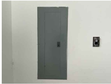
Main Service Panel Manufacturer: General Electric
