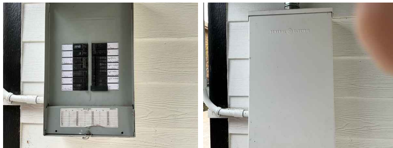
Sub-Panel Manufacturer: General Electric
