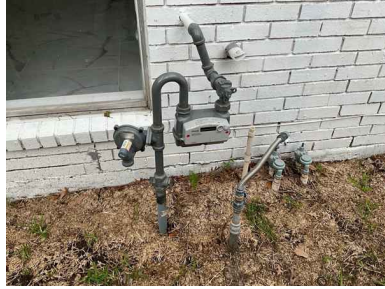
Type of Gas Distribution Piping: Polybutylene, Stainless Steel
