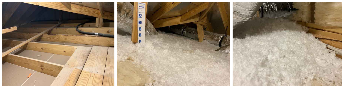
Viewed From: Decked portion of the attic due to amount of insulation Approximate Depth Of Insulation: 4"-6"
